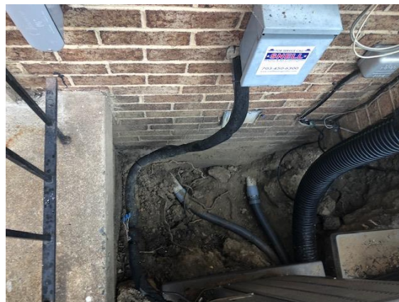
New electrical lines were placed in PVC conduit which extend from the meter island through the foundation to each unit's electrical panel.
