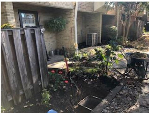
To fully resolve recurrent flooding at 1701 Kenwood, the drainage system was tested and a drainbox relocated after coordination with the unit owner and residents.
