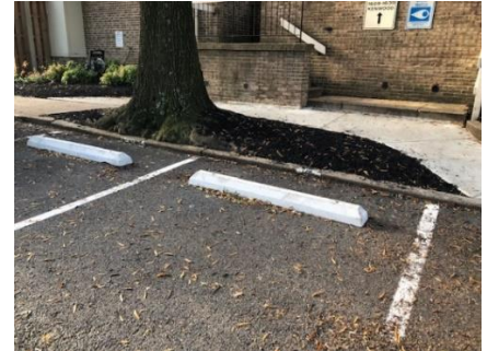
View of barely visible parking numbers painted on too-short curbs
