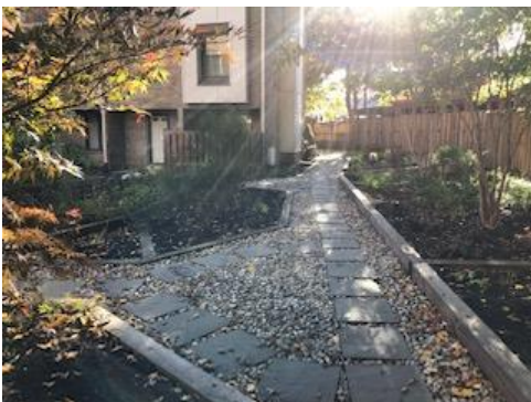
After: A complete stormwater drainage system has since been installed and is covered by aesthetic landscaping.
