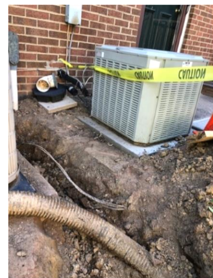
As shown above, the original electrical line was buried directly in the ground and not at the minimum 24" depth.
