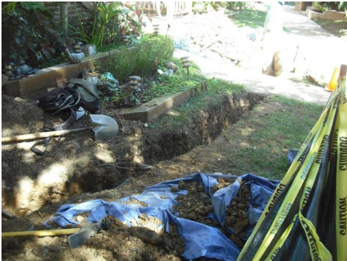
Part of the trench dug for 1750 Dogwood Drive remains to facilitate the replacement of other units' electrical lines, using the same trench.
