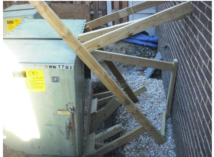
The area under the transformer has been repeatedly dug up for multiple electrical issues over the years, and has been stabilized for completion of The Dogwood Dig.
