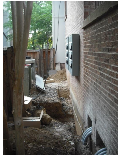
Entry holes had to be cut into the retaining walls on the side of each building, as pictured on the bottom right.
