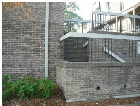
The originally planned location for new meters would have required cutting through and underneath the stairs.
