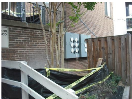
View of fence with section removed to install new meters on the wall; the fence will have to be rebuilt.
