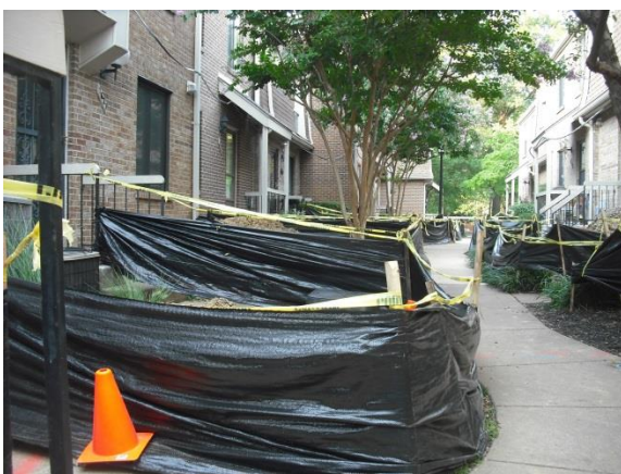
Protective barriers were installed around the trenching in front of each unit as a safety measure.
