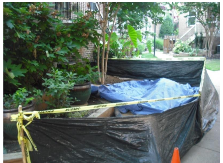
View from 1728 Dogwood Dr of protective barrier around the trench dug in front of 1748-1750 Dogwood Dr.
