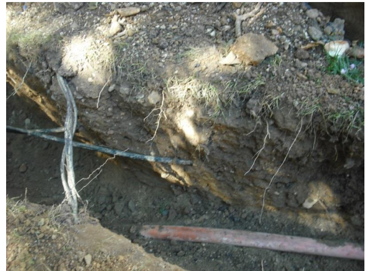
Note the electrical wires buried only inches below ground.
