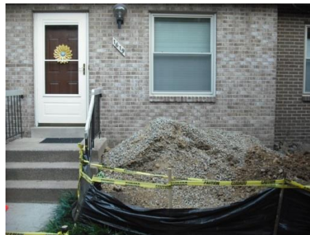
Piles of rocky subsoil were stored in front of several units while electric supply lines were replaced.
