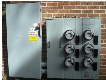
In late August, the City changed code requirements for the project, with the mandate that shutdown boxes (on the left) be added.
