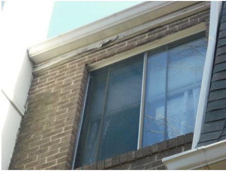
Rotting fascia board above the window.
