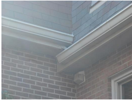
Damaged fascia board above the gutter.
