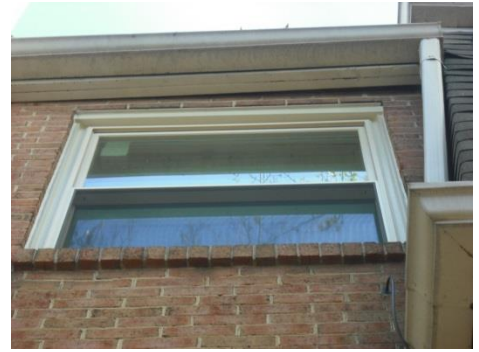
Fascia board warped away from building.
